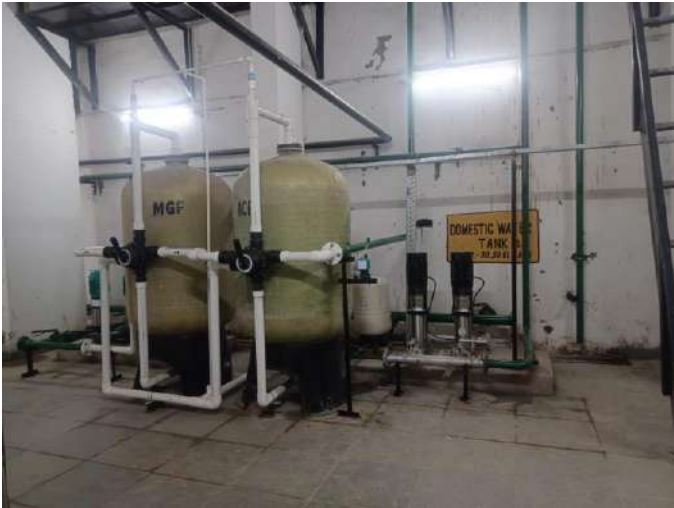
WATER SOFTENER PLANT
