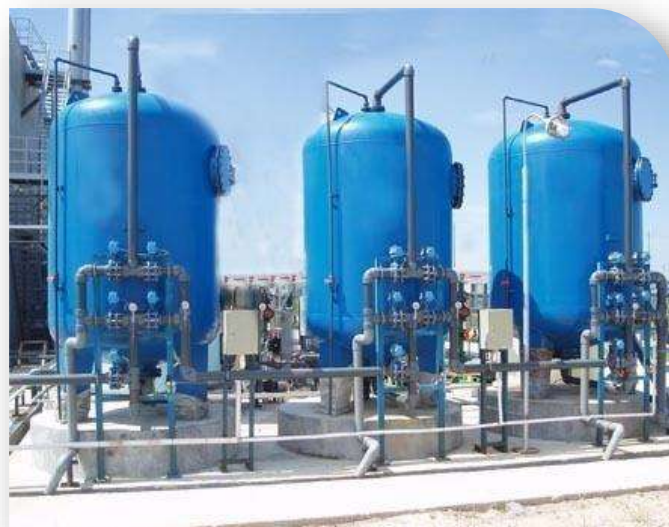
WATER SOFTENER PLANT
