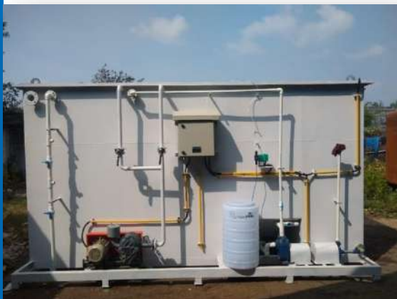
WATER TREATMENT PLANT
