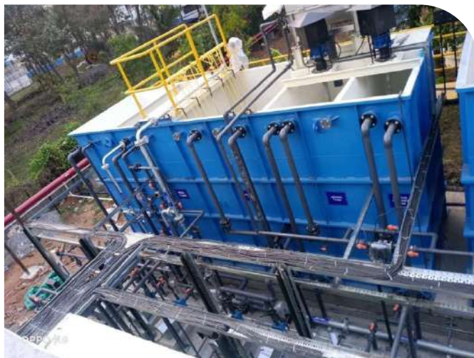
SEWAGE TREATMENT PLANT
