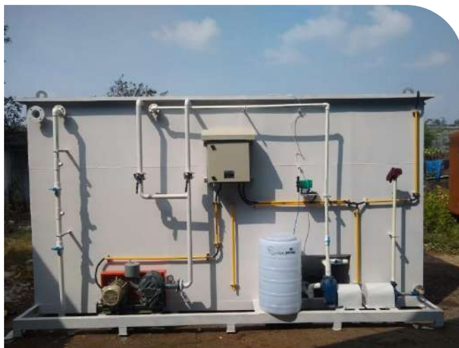
SEWAGE TREATMENT PLANT
