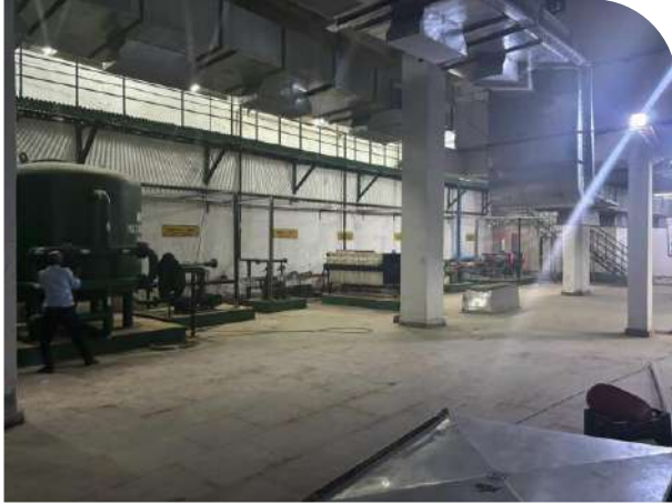
SEWAGE TREATMENT PLANT
