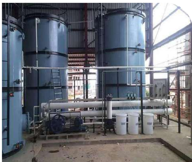
ZERO LIQUID DISCHARGE PLANT
