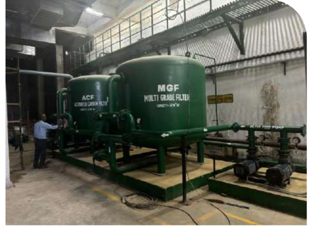
SEWAGE TREATMENT PLANT
