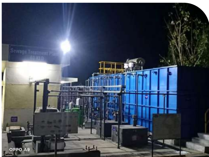
SEWAGE TREATMENT PLANT
